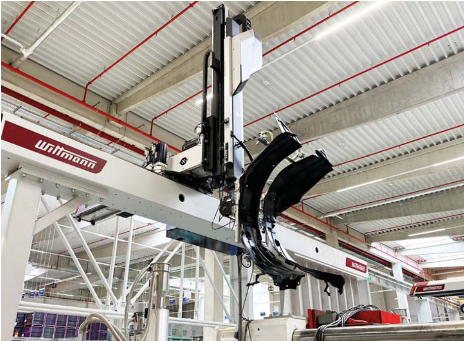
The new injection molding production operates with highly automated systems. All injection molding machines are equipped with linear robots from WITTMANN's W and WX series.
