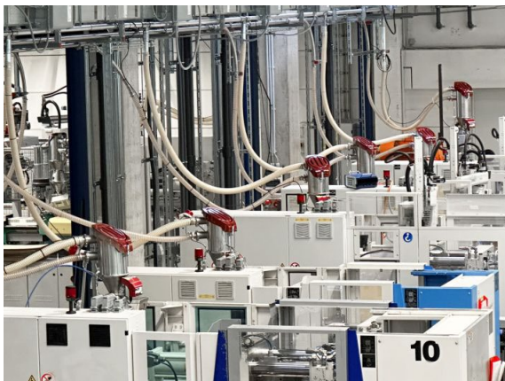
The granulate is transported inside a closed system. Feedmax Clean material loaders are also used. In this way, dust generation is reliably prevented.
