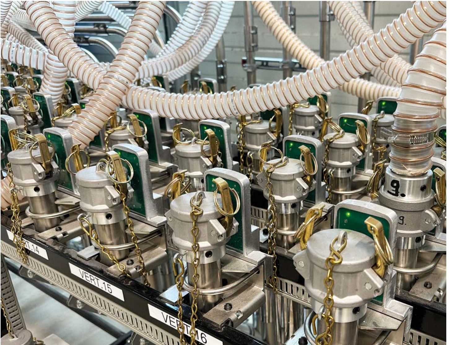
The new coupling station still leaves room for further growth.
