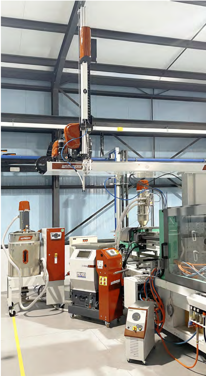
Automation and peripheral equipment for one of the AB Inject injection molding machines: W821 robot, Drymax material dryer, Feedmax S3 net material loaders, Tempro basic C temperature controller, and S-Max 3 granulator.
