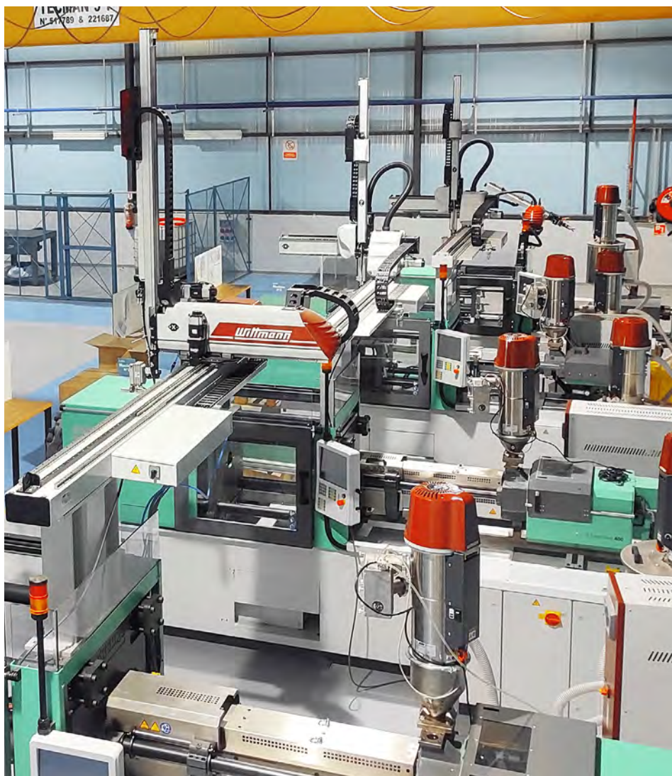
A view of the WITTMANN peripherals and robots installed on and next to AB Inject's injection molding machines.
