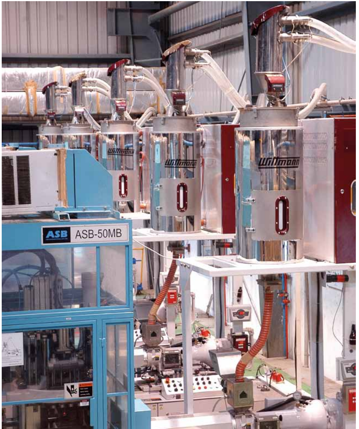
A view of the central drying and conveying system at Swashtik Preforms based in Pondicherry, India. The entire system is dedicated to PET processing.
