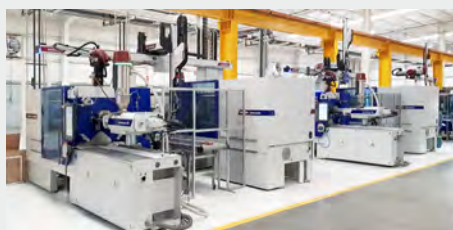
Page 12: Unique working cell solution for ISGO causing a furor in Mexiko.
