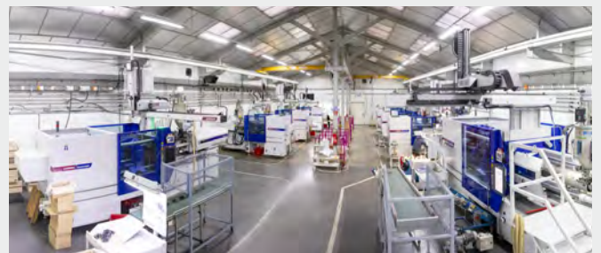
Page 8: PLASTIFAL, France, saves money and takes care of the environment, assisted by WITTMANN.
