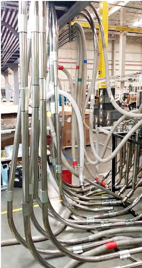
Conveying system detail before WITTMANN BATTENFELD do Brasil started working.
