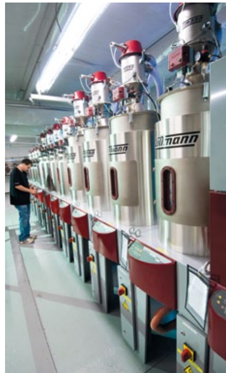
Centralized materials drying and conveying with this WITTMANN system on a mezzanine is another important component of automation at Vision Technical Molding.
