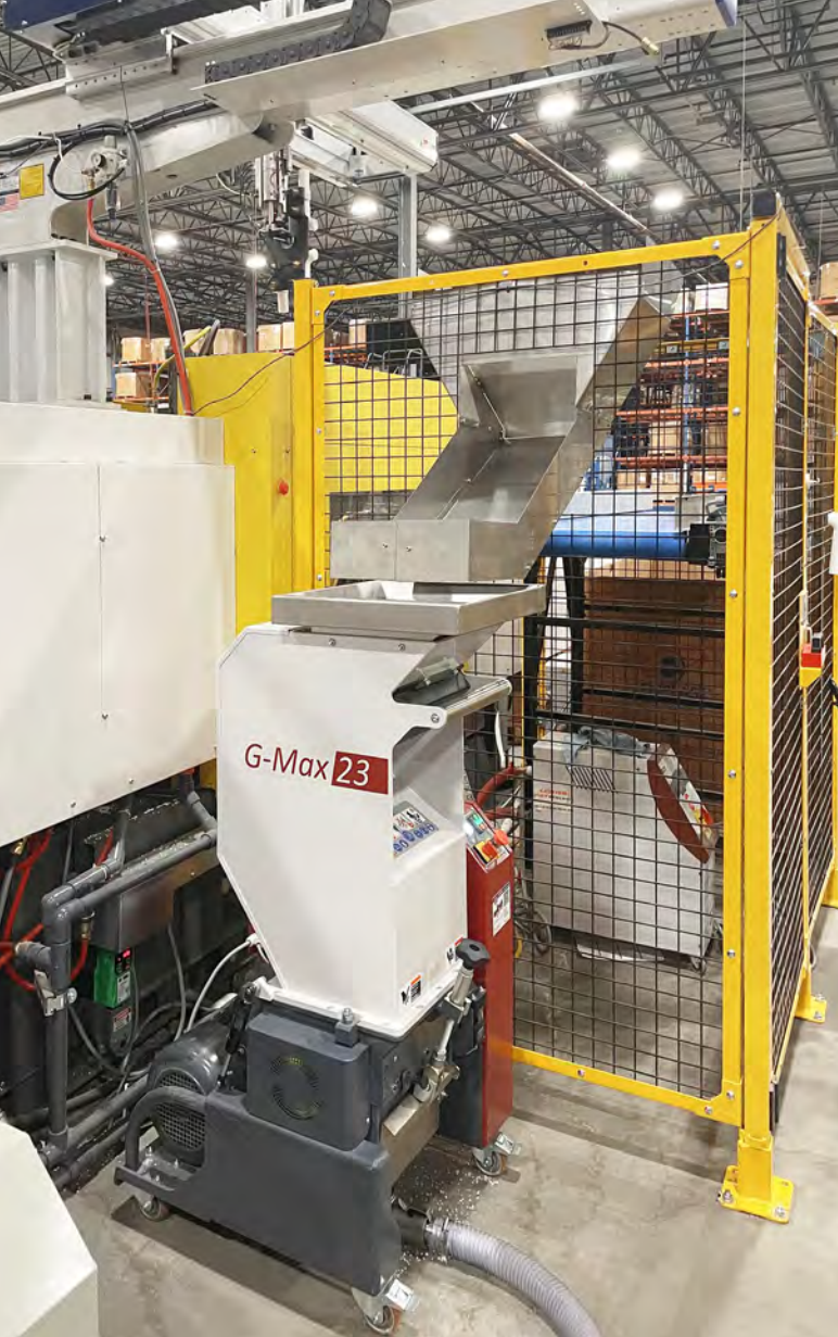
G-Max 23 beside-the-press granulator at the Keeney plant in Winchester, New Hampshire.
