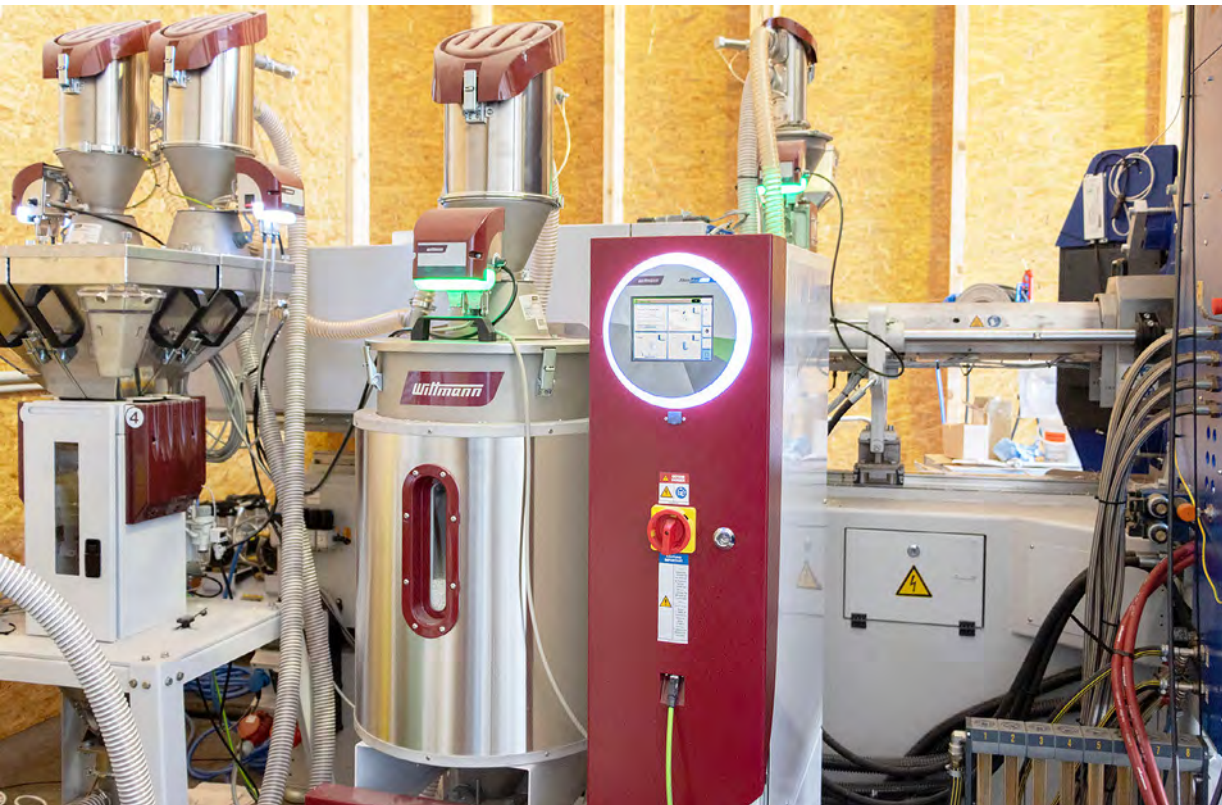
Metering, material loading and drying technology from WITTMANN, installed at ANA-U.
