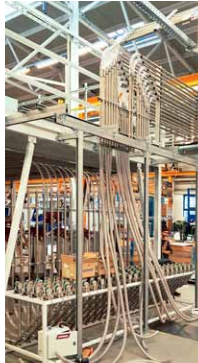
Views of the piping of WAREMA PT's material conveying system.
