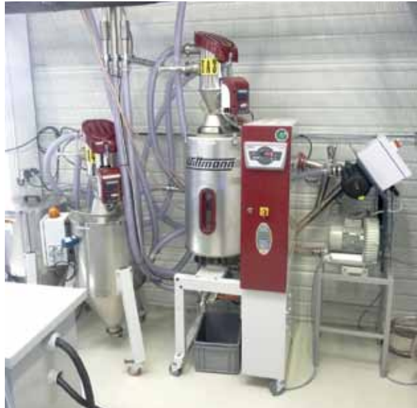
The NICOMATIC installations
